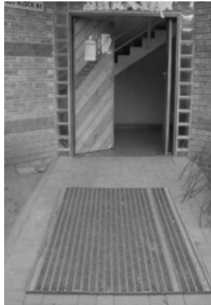
Figure 16: Uneven mat at hostel entrance
